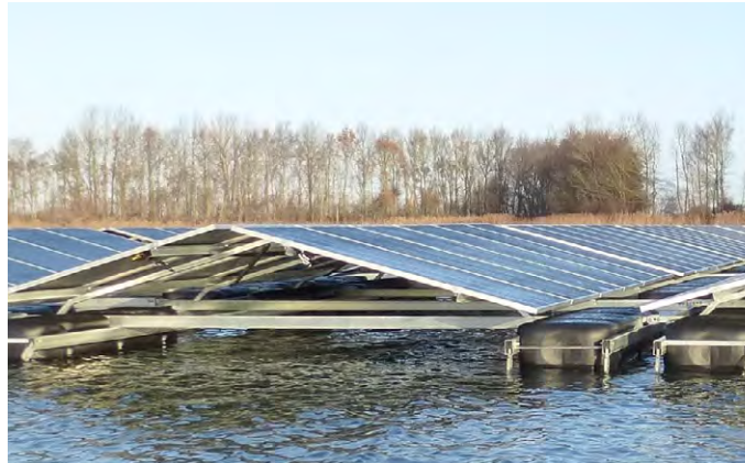
Floating solar power plant utilising Magnelis™, Netherlands
