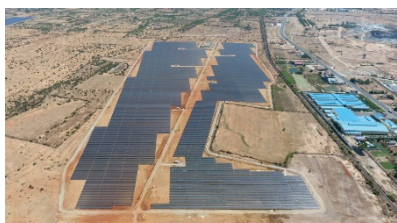
Industrial Solar Power System
