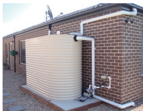
A 4,000-liter rainwater storage tank
