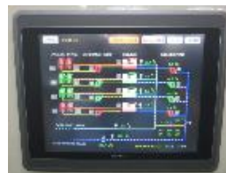
Air conditioning equipment control panel
