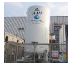
Nitrogen supply system
