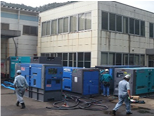
Disaster recovery support (lending electric generators)
