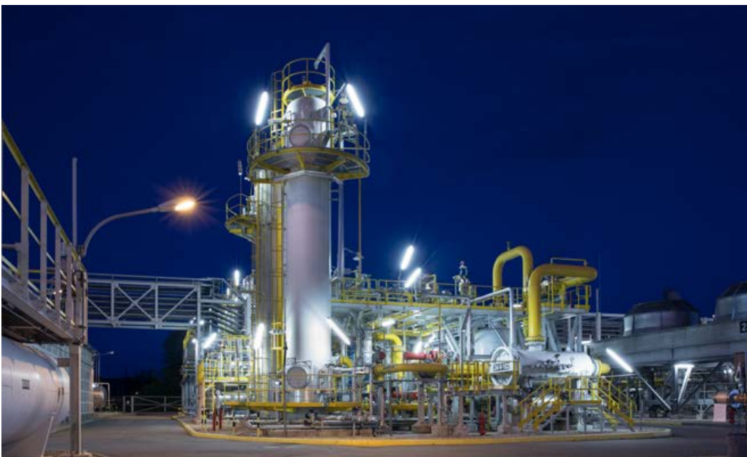
Hurezani – gas treatment station
