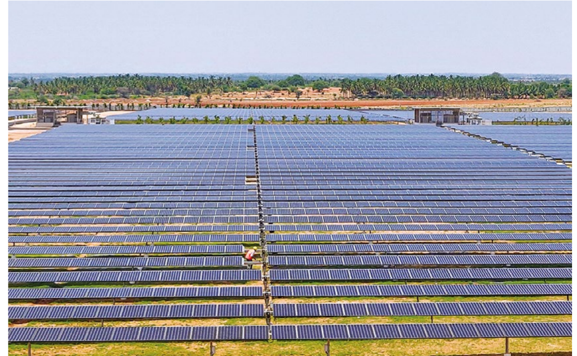
40 MW solar plant in Sira, Karnataka
