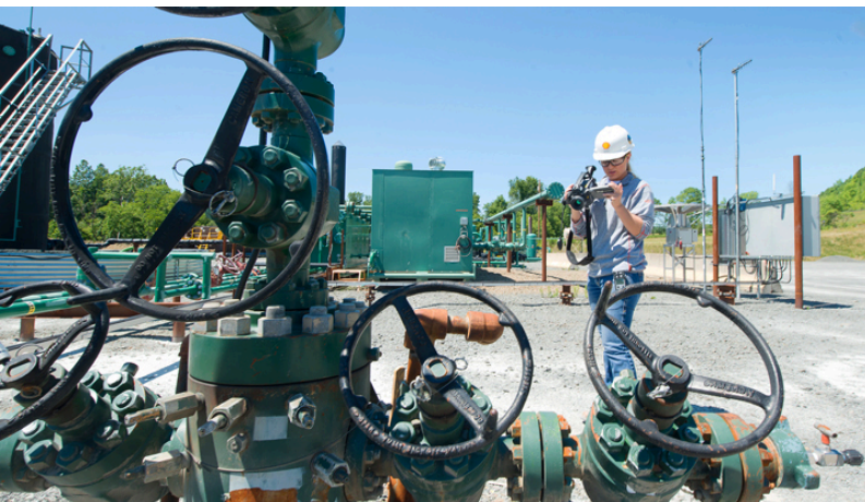
A Shell employee inspects equipment for potential methane leaks at a facility in Pennsylvania, USA.
