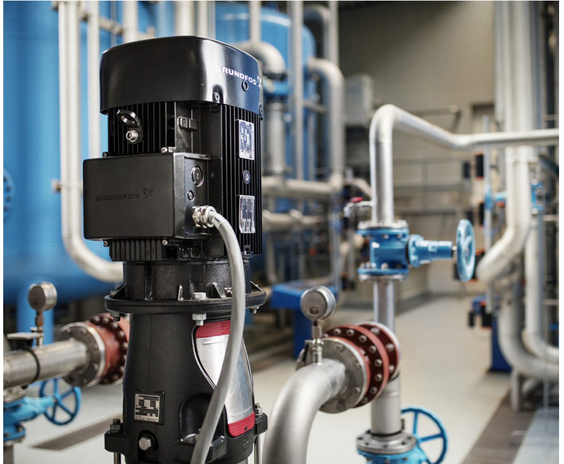
The Grundfos CR-95 multistage pump at WWSB in Oberwart, Austria
