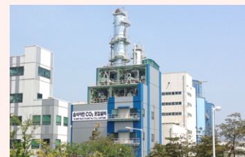
Boryeong Thermal Power 10MW Wet-Scrubbing CO 2 Capture Plant
