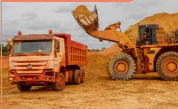
EGTF, the Malian construction company, loading topsoil at the Viper Satellite pit near Morila.
