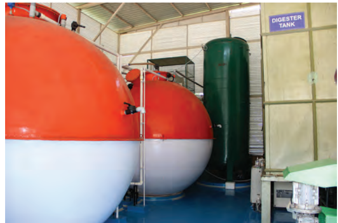
Biogas plant at Infosys Hyderabad campus
