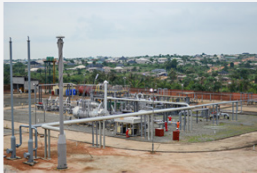
The Agbara/Ota pressure reduction and metering station in Ogun State, where new production facilities were added in 2018.
