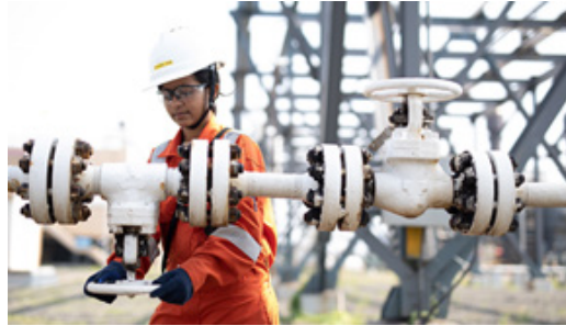
Shell operates a liquefied natural gas regasification terminal in Hazira on the west coast of India.
