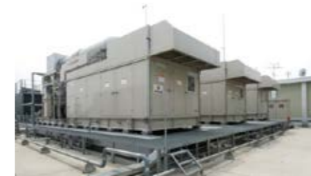
Aeon's private power generators
