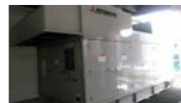
Gas-engine generator at Aeon Mall Makuhari New City
