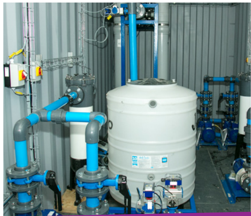
Installation of our reverse osmosis desalination plant
