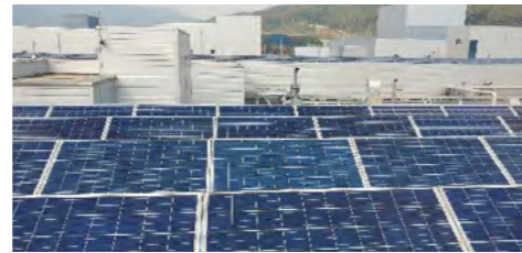
Jeungpyeong solar power plant
