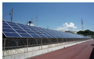
Solar power plant in Hidamari-no-Oka
