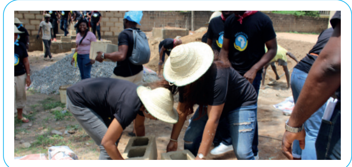
Employees of Union Bank, helping in the construction of modern toilets in a government-owned school
