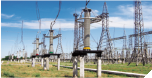
△ Kazakhstan Power Transmission and Substation EPC Project
