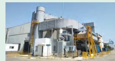
A high-efficiency VOC processing facility.
