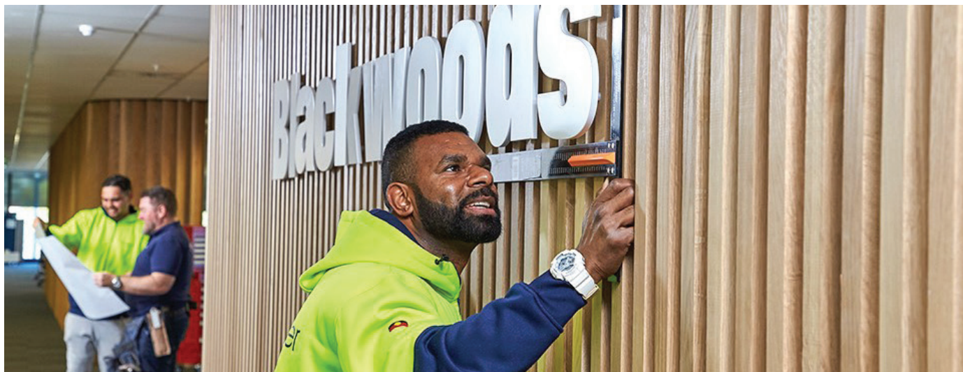
Mark Mosby, one of the tradesmen employed by Blackwoods' contractor "The Builder-Sydney", puts finishing touches to the new Blackwoods Internal Sales office in NSW.
