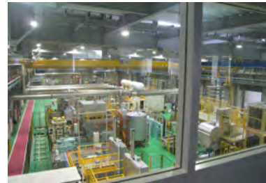
Unattended area viewed from manned area (production facility)
