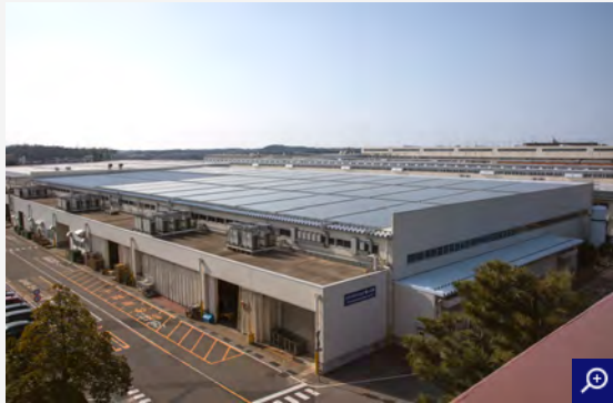
Solar panels on the roof
