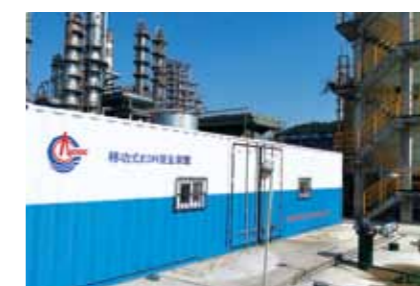
◀ Field operation of electrochemical water quality stabilization demonstration device
