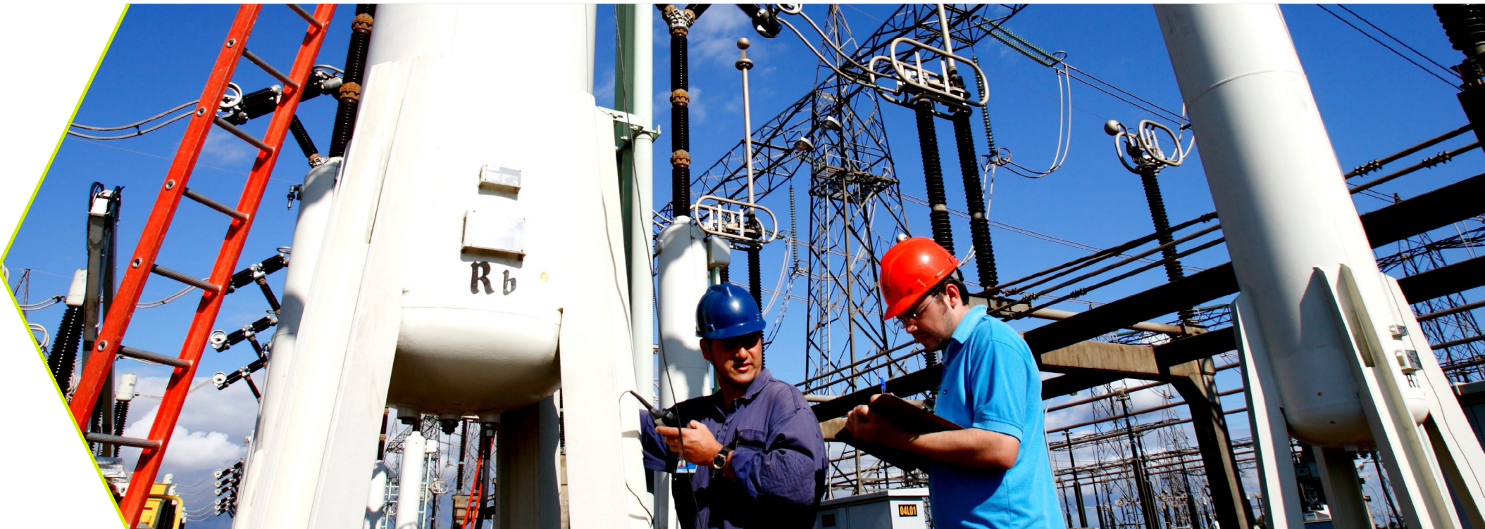
Substation in Itaipu – Itaipu Binational/Caio Coronel
