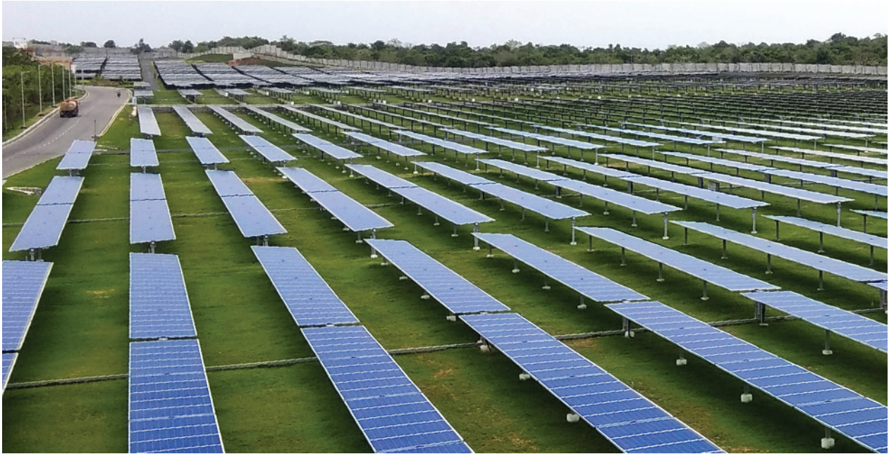
Our 6.6 MW-capacity solar farm in the Hyderabad Pocharam campus
