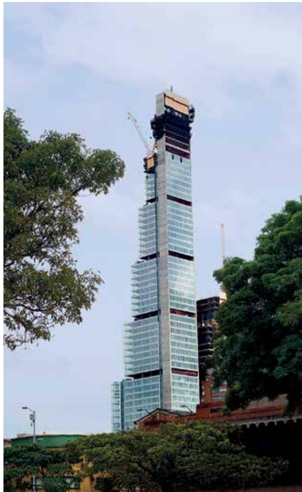
Infrastructure built with Argos: BD Bacatá, Bogotá, Colombia
