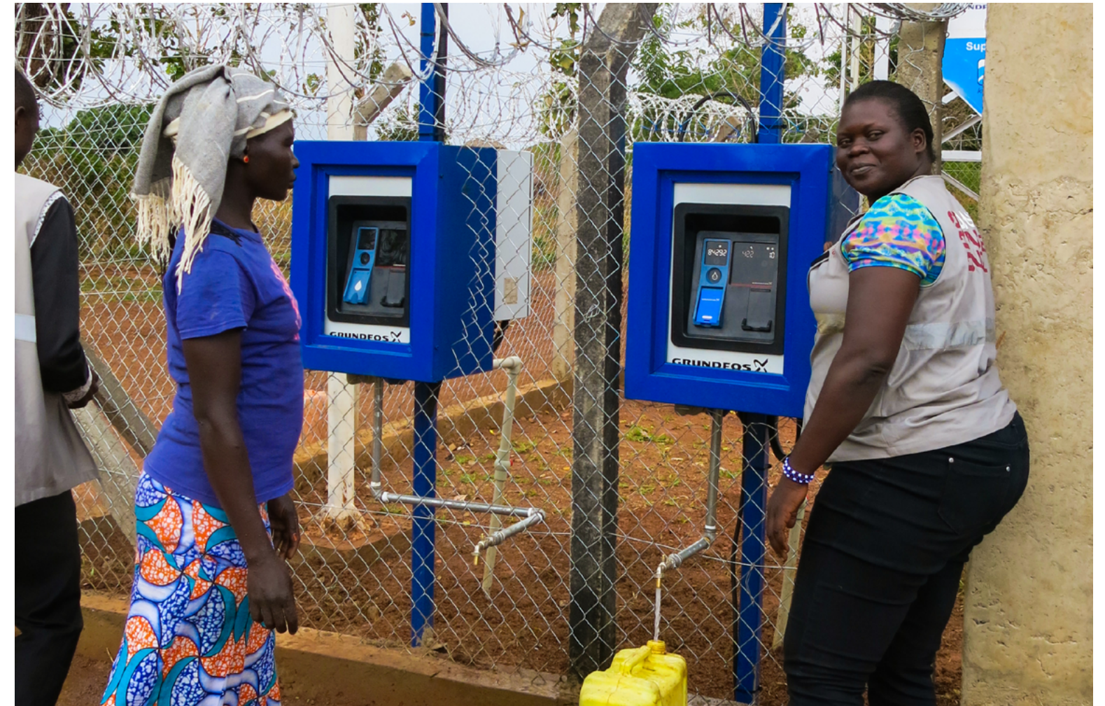
The first water solutions for the Bidi Bidi refugee camp in Uganda were successfully installed
