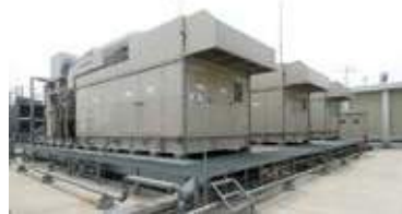
Private power generation equipment installation
