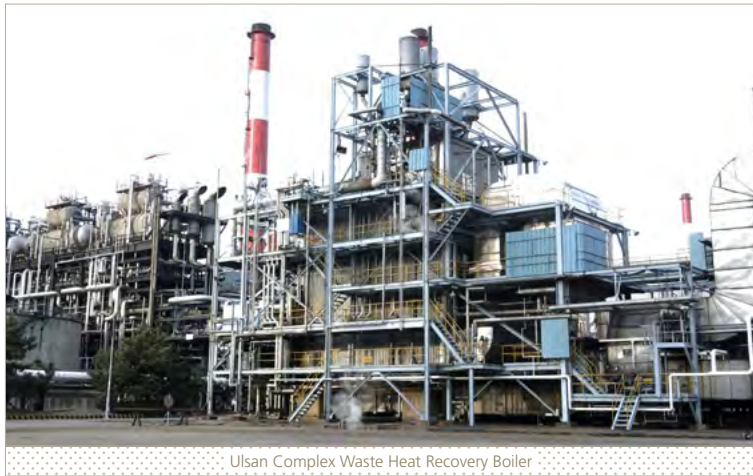
Ulsan Complex Waste Heat Recovery Boiler
