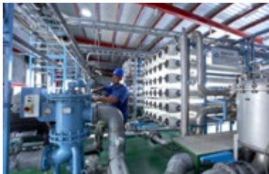
A seawater desalination system.
