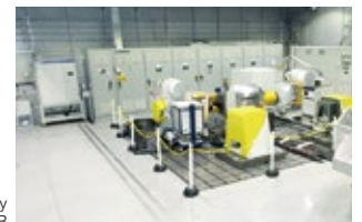
The electric motor testing facility in HORIBA BIWAKO E-HARBOR
