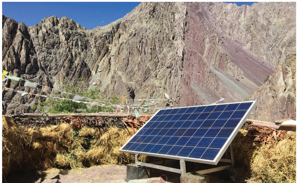
The solar grid project with a total capacity of 24 KW in progress
