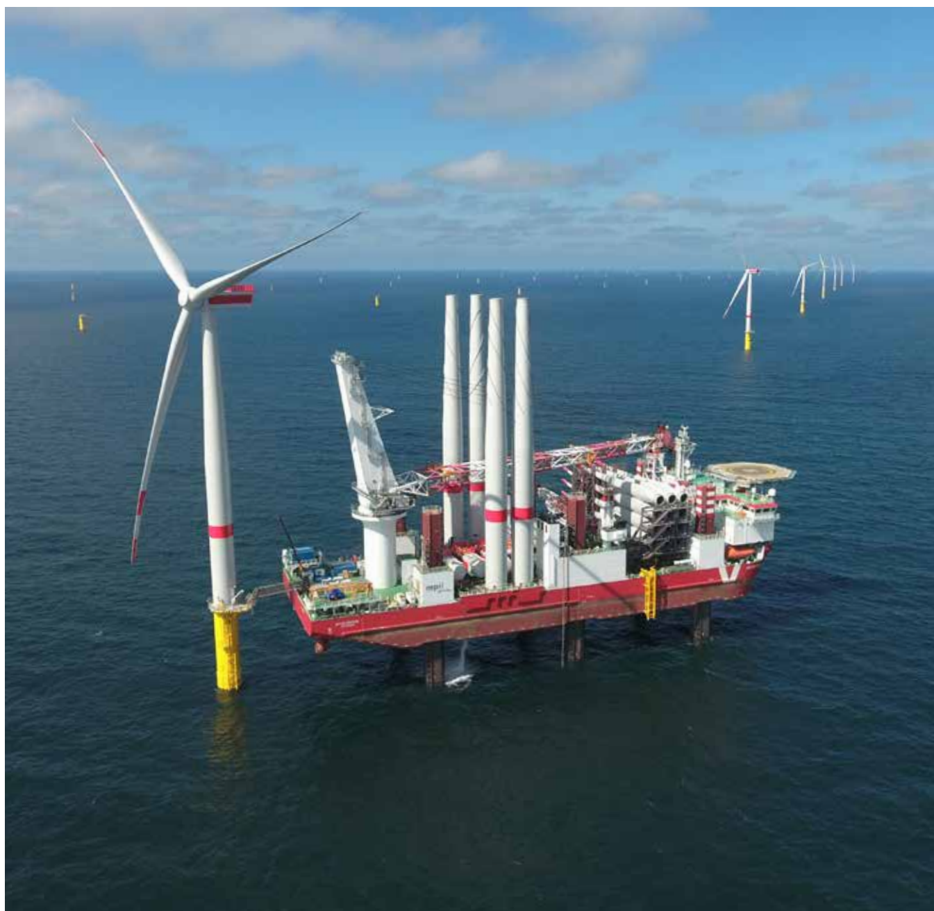
Our Sandbank (288 MW) offshore wind farm in Germany began generating power in September 2016 and was delivering at full capacity in early 2017, three months ahead of schedule.
