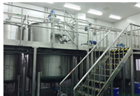
Enhanced facilities (tanks)
