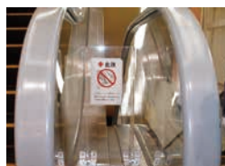
Safety Measures for Escalators
