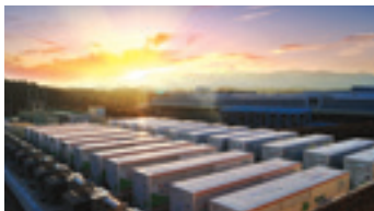
ESS in Gyeongsan Substation
