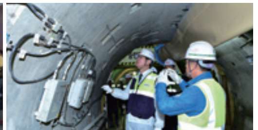
Site Inspection of Electric Equipment during the Extensive Diagnosis of National Security
