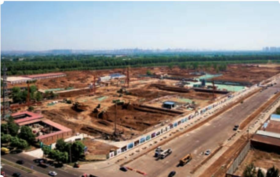
Land development project for shanty town transformation in Tongzhou financed by CDB Beijing. After completion, the project will move 400,000 people away from the capital. It is of great significance in realizing regional plan and accelerating the movement of non-capital functions of Beijing's downtown.
