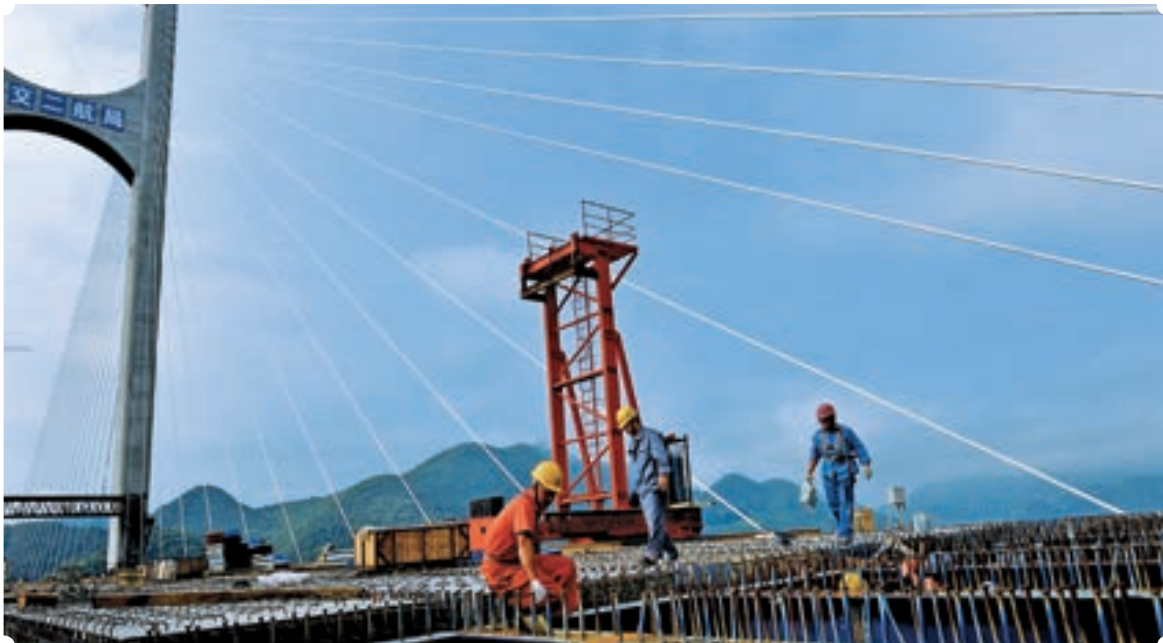
Zhingjian River Bridge project of the Enshi-Laifeng expressway is a kingpin project in the poverty relief program. CDB Hubei formed two consortia, one with 5.6 billion yuan and the other, 4.6 billion yuan to finance the project. When completed, the project will remove the bottleneck in between the Wuling area and Shanghai and Guangdong.
