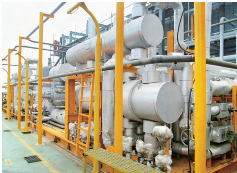
▲ Natural gas processing facility in WHPA platform of “Bozhong 26-3” oilfield
