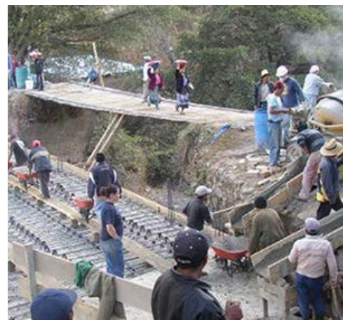
Construction of a 45-meter-long pedestrian footbridge to serve the residents of La Conga, Panama; this bridge was built by 11 CH2M employee volunteers, in collaboration with Bridges to Prosperity and the residents of La Conga.
