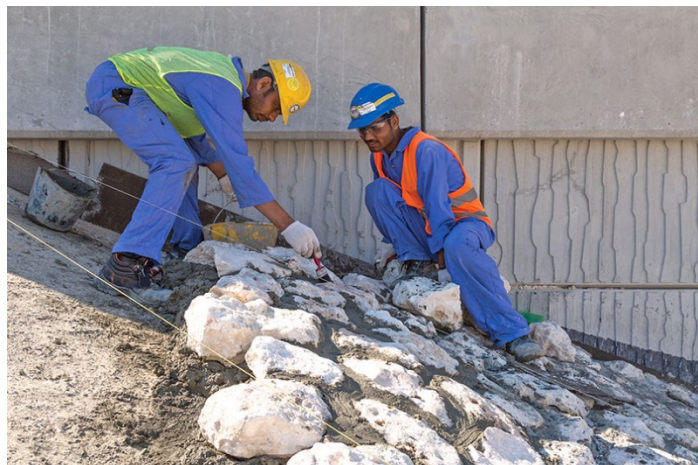
Workers on a CH2M Foundation project in Nicaragua, building a concrete foundation for a holding tank on a large hill
