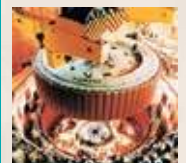
Siemens installs the first of 18 Itaipu generator rotors, with a power of 823.6 MVA.
