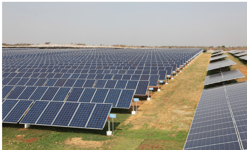
Solar power plant set up in the Hyderabad (SEZ) campus
