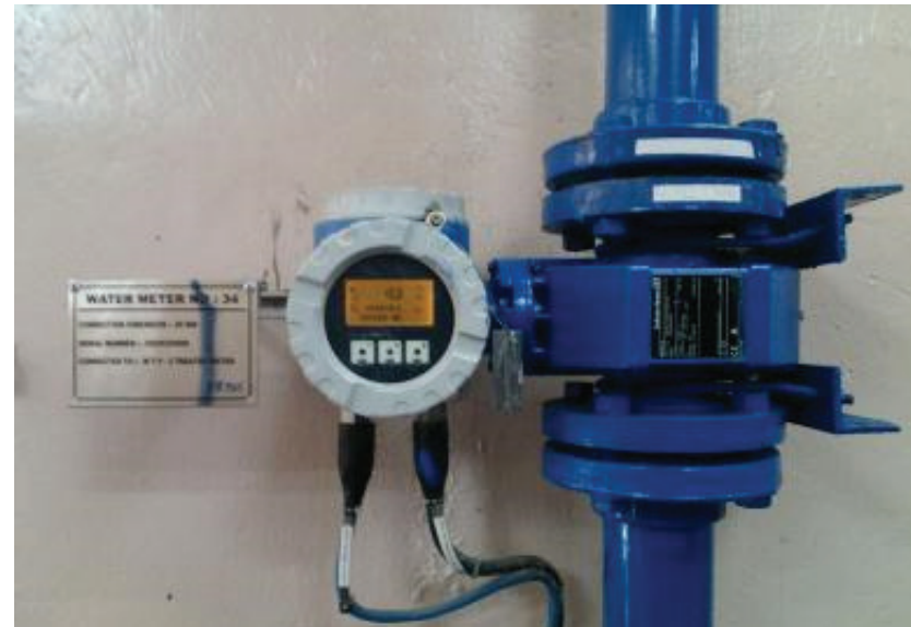
Smart water meter for online monitoring of water consumption
