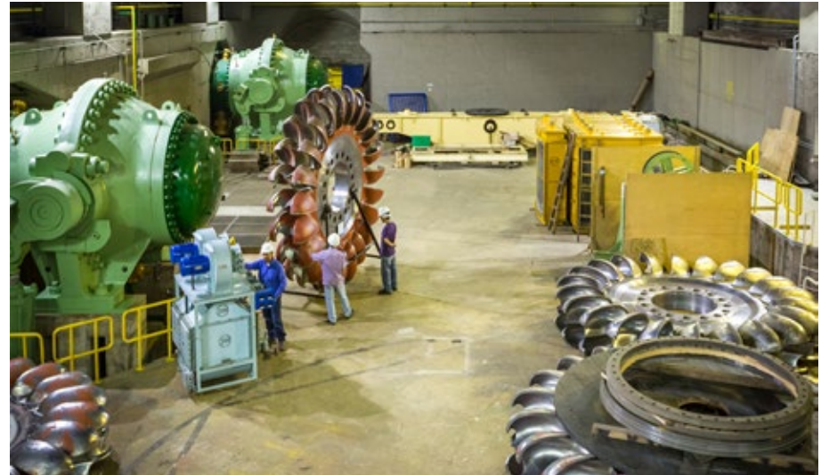
Machine station. San Carlos Hydroelectric Power Plant
