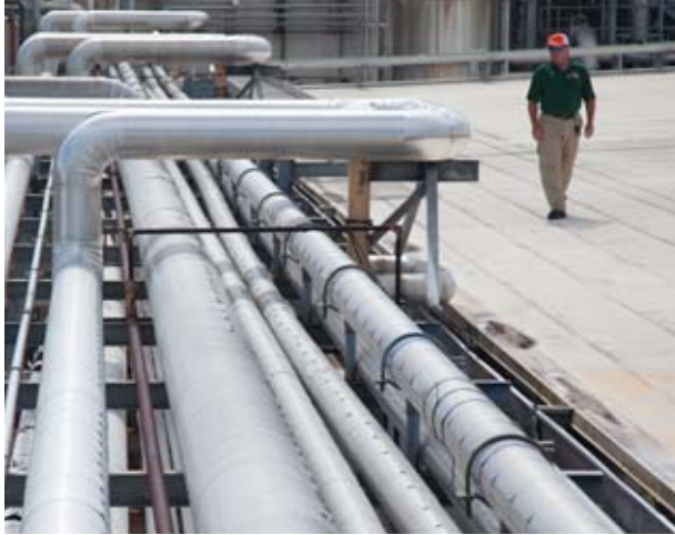
A cogeneration facility where we convert local landfill gas to energy at the Tropicana plant in Ft. Pierce, Florida
