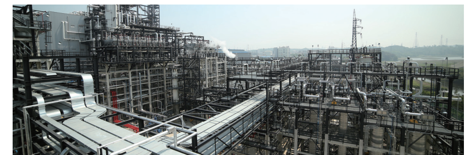
SK Global Chemical's Nexlene Production Plant
