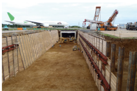
Inclined-braceless excavation support (Narita Kinone Tunnel No. 2 installation project, Narita International Airport)
