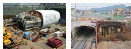
A shield tunneling machine beginning the tunnel above ground (left) and arriving at the other end of the tunnel (right)
