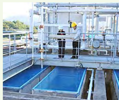
Tank in which chemicals are decomposed using microorganisms
