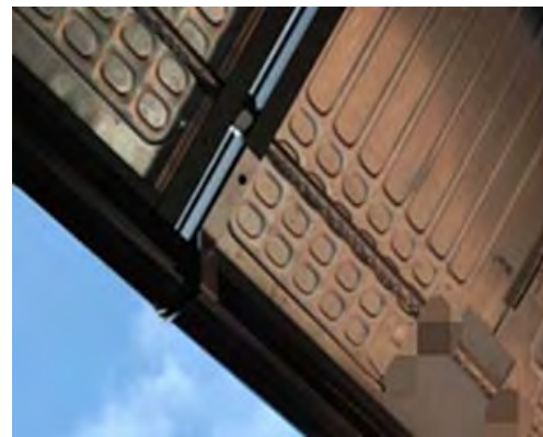
PV-thermal system (drain pipe on the underside of a solar module)
