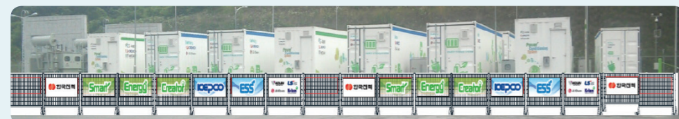
ESS for Frequency Adjustment(Seo-Anseong Substation)
