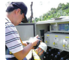
Diagnosing safety in facilities
