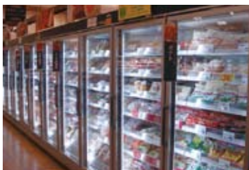
Refrigerator showcase using natural refrigerant (CO 2 ) installed at Aeon Mall Makuhari New City Store
