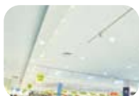
Transition to LED lighting
