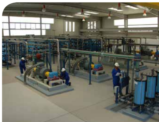
Metito Seawater Reverse Osmosis Plant in Marsa Alam-Egypt
