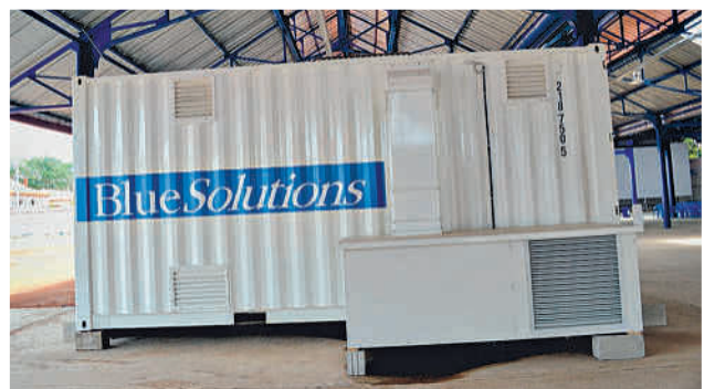
Blue Solutions battery via stationary application.
