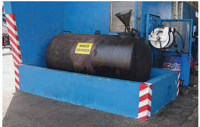
Waste oil storage tank – Dakar (Senegal).
